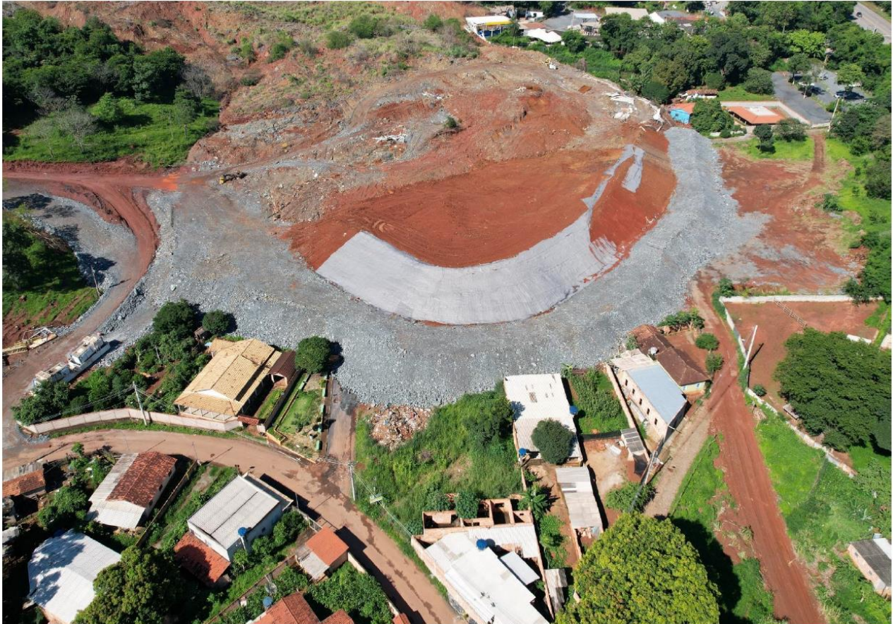
Figure 3: The 400-metre-long containment barrier built around the slumped material to prevent any further movement and protect the adjacent community.
