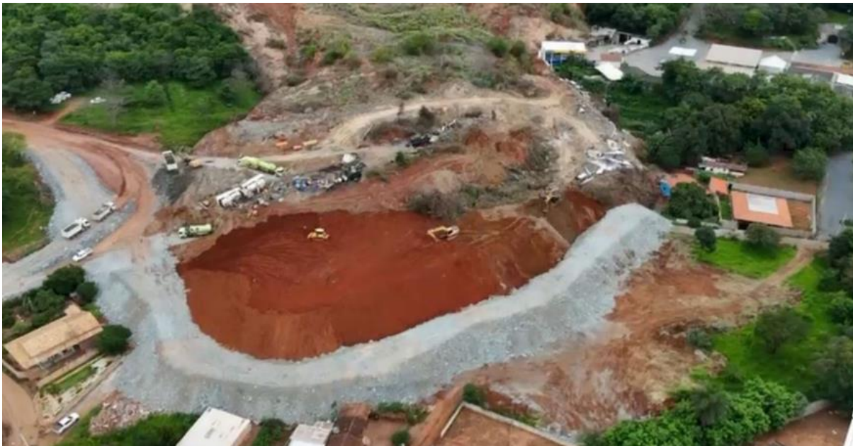
FIGURE 1 – The 400-metre-long containment barrier built around the slumped material to prevent any further movement and protect the adjacent community.
